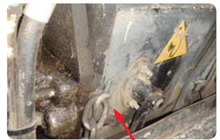
Manufacturers provided locking device inoperative and chain used with a 'D' link to prevent accidental extension.
