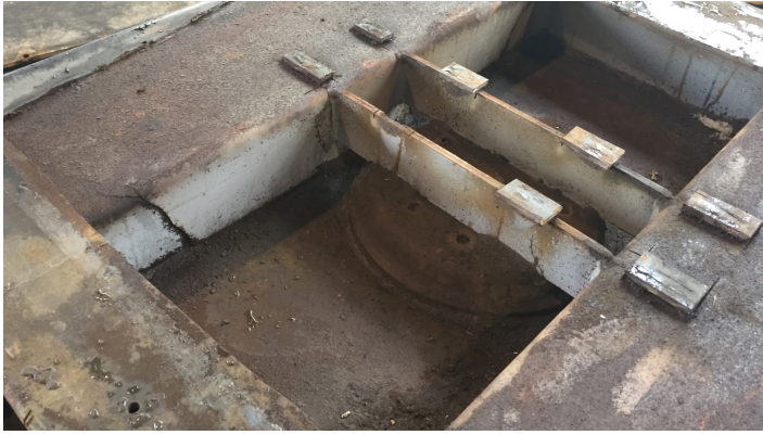
A closer inspection reveals a serious structural failure of the cross-member
