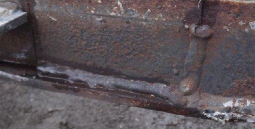
This skidplate has signs of previous repair and fresh cracks. It should not be used and it should be referred to an HVSC.
