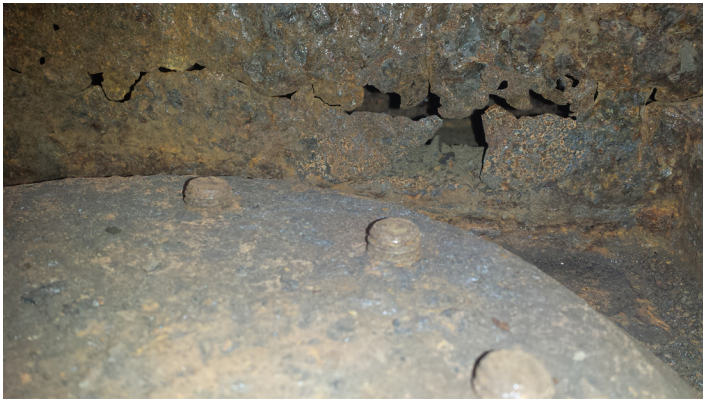
A closer inspection reveals corrosion around the skid plate support structure
